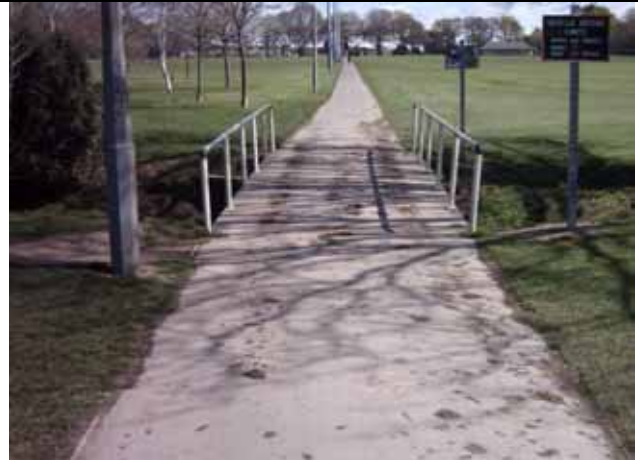
Figure 17: Bridge with minimal rails and no approach barriers
