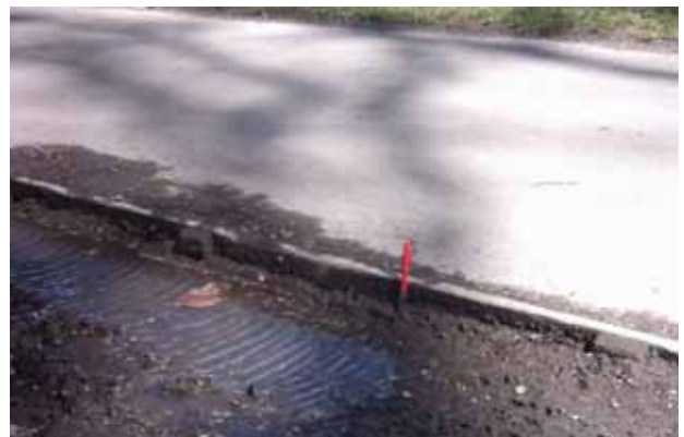
Figure 15: Red pen showing dangerous drop
